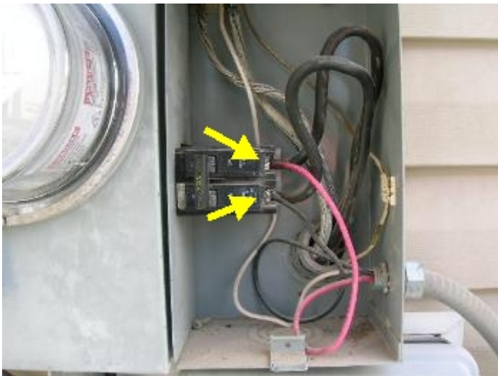
There are two wires to one breaker. This is double tapping and not recommended. There is one breaker in the sub panel and the main breaker in the main box. Recommend repair by a licensed contractor.
