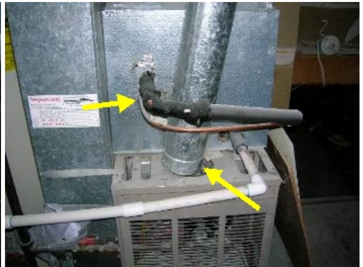
The vent is disconnected and the insulation should be redone on part of the A/C line.
