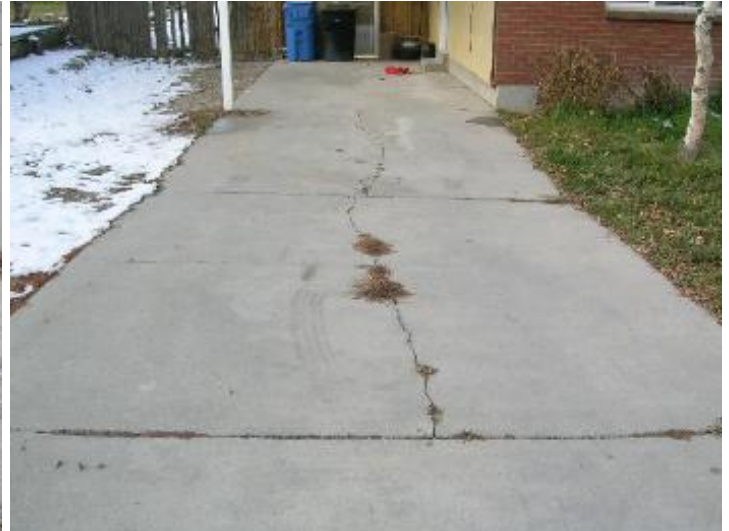
Common cracks upto 1/4" were found in the driveway at the time of the inspection.
