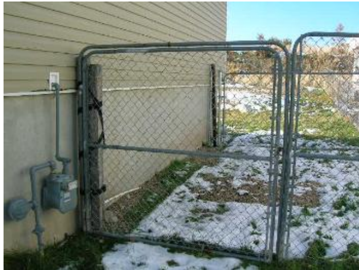
Small hole present on the west side of the house.
