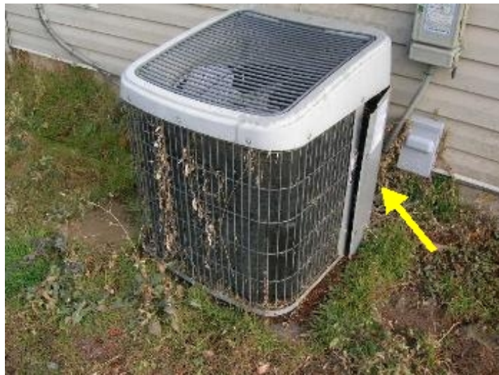
Part of the panel is loose on the unit.
