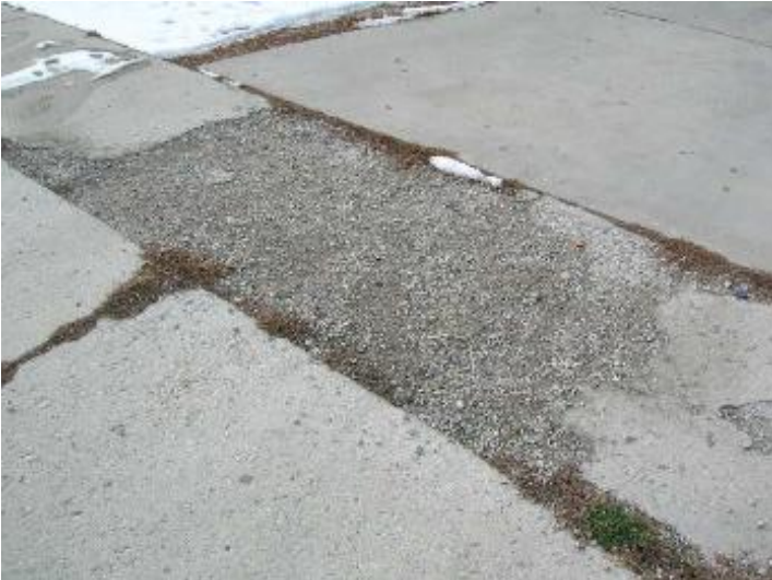
Deterioration on the front sidewalk.
