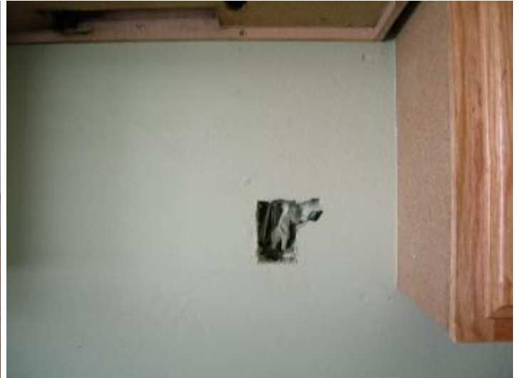
There are electrical wires in the wall without an electrical box. This is not recommended.
