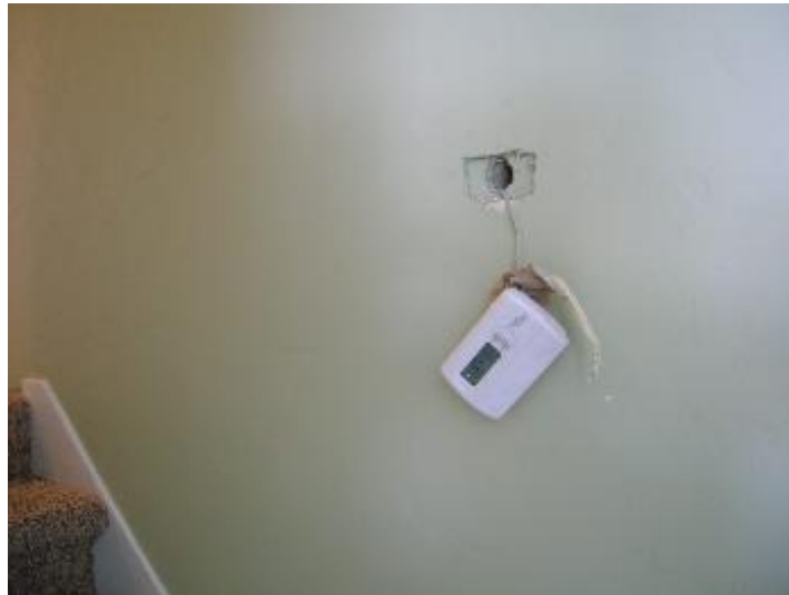
loose on wall
