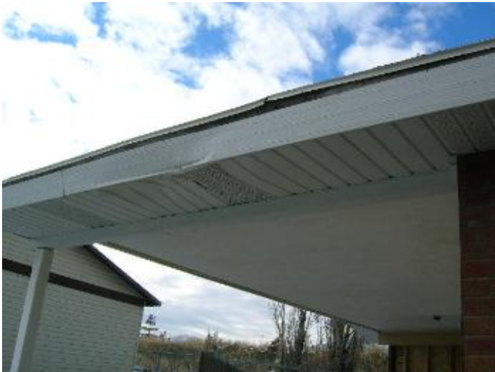
There is damage on the facia and soffit of the carport.
