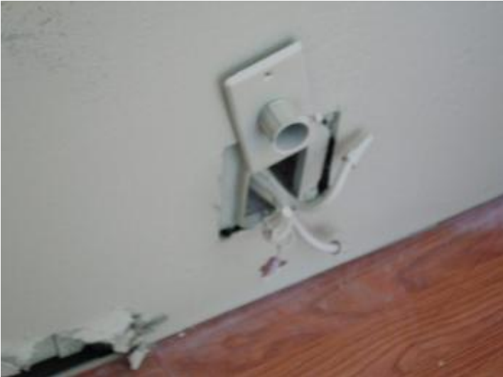
The 220 volt outlet in the kitchen has caps on the wires and no plug installed.
