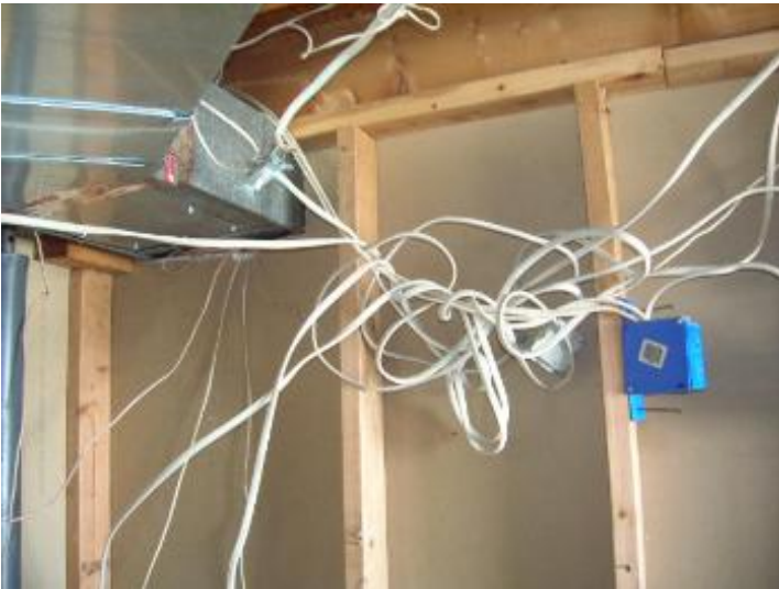
There are many wires and exposed wiring that need to be secured in the furnace area.
