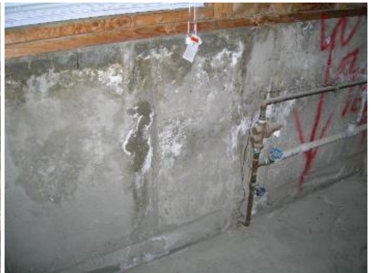
There is moisture stains present on the foundation wall in the furnace area.
