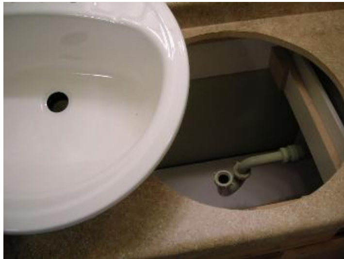
The sink in the main bathroom is not installed.
