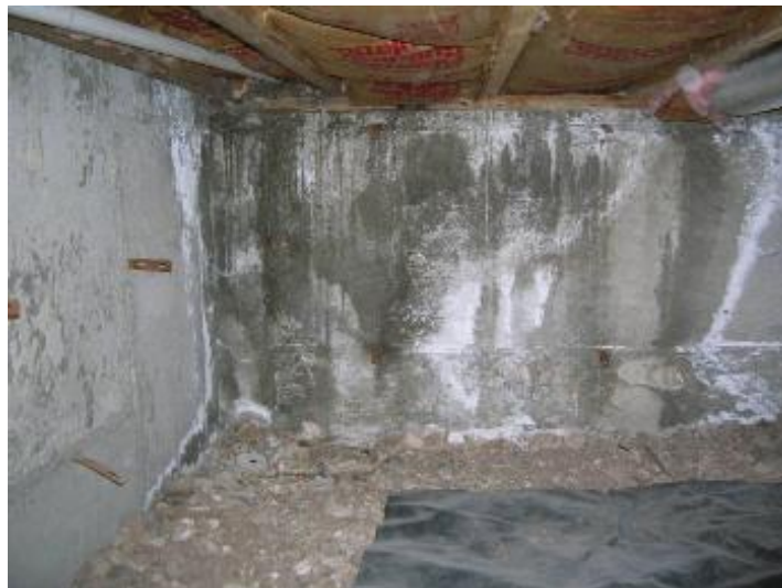
There is moisture present on the foundation wall in the crawlspace at the SW corner. Recommend further evaluation by a licensed contractor.
