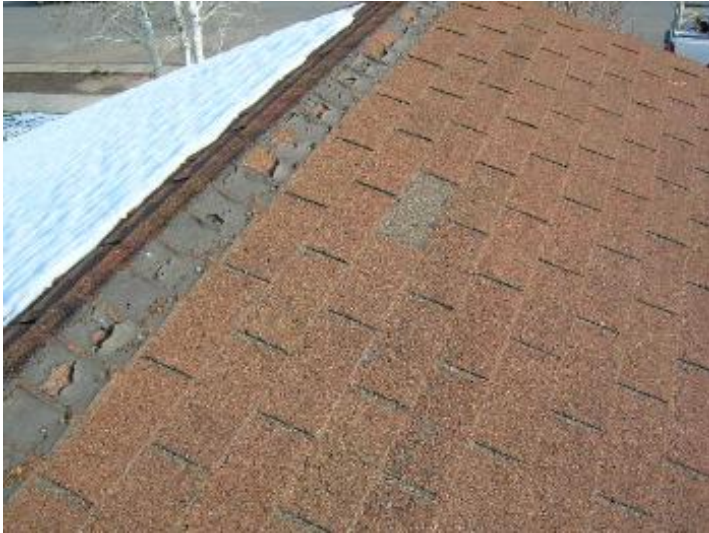
deteriorated shingles at ridge cap
