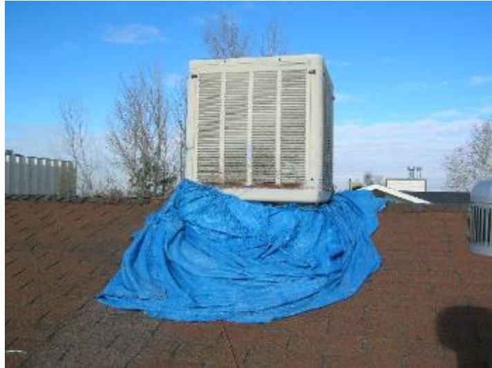
The cover has come loose of the swamp cooler.
