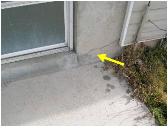
There is a common crack on the foundation.
