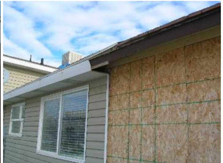
The soffits are not finished on the west side of the carport.
