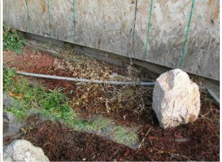
There is wood on the bottom of the carport wall that is in contact with the dirt. This is not recommended.
