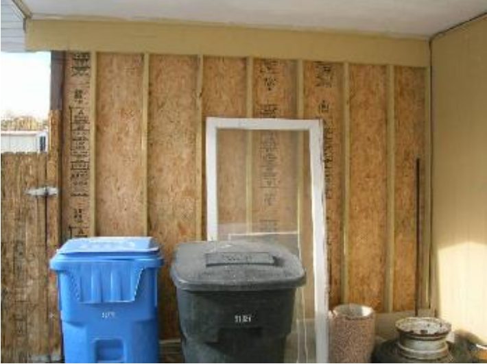
The rear wall in the carport is not finished.
