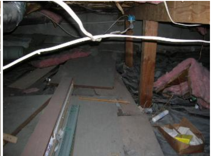
The electric wiring is not properly secured in the crawlspace.
